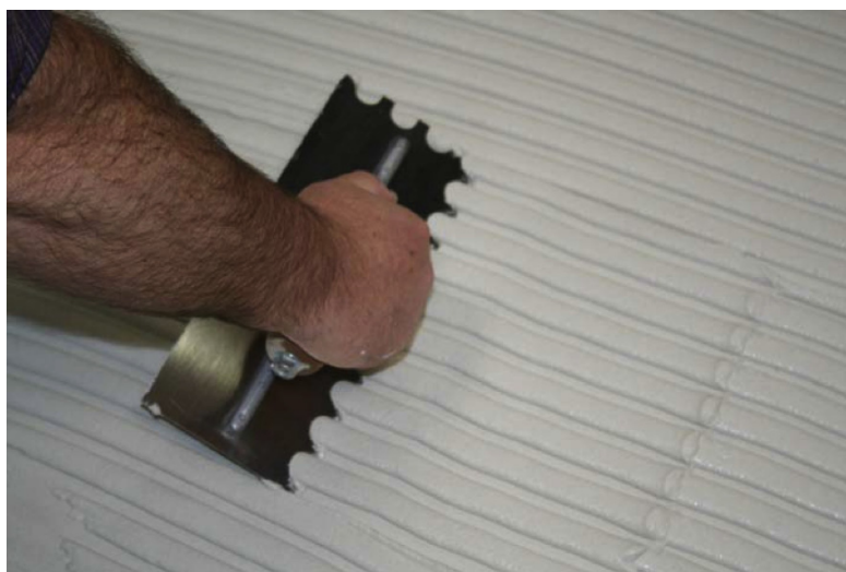
Picture 1.2 – 18 mm loop notch trowel with a medium bed adhesive used for large format tiles or stones. Trowel thin set adhesive in one direction holding trowel at a 45 degree angle. Notice the full ribbons of adhesive that left behind.
