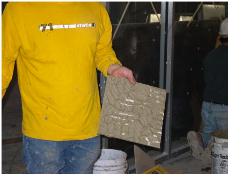
Picture 1.4 – Ceramic tile removed during the installation to verify proper coverage is being attained. Notice the lower right hand corner of the tile is lacking coverage. This will undoubtedly lead to a cracked tile.
