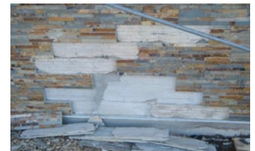
Delamination of Stone
