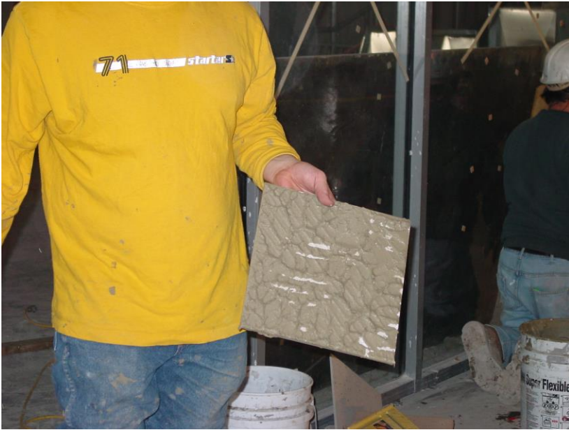
Picture 1.4 – Ceramic tile removed during the installation to verify proper coverage is being attained. Notice the lower right hand corner of the tile is lacking coverage. This will undoubtedly lead to a cracked tile.
