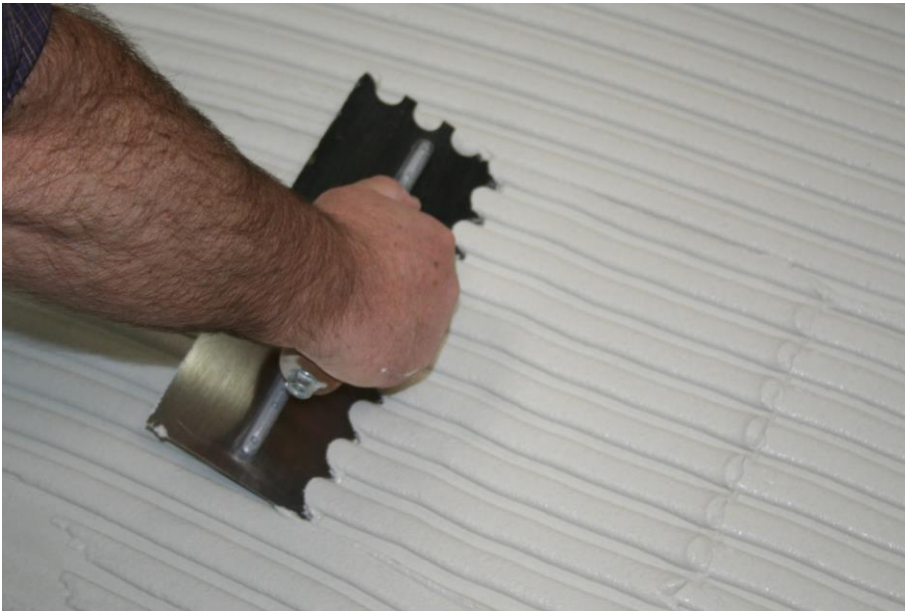
Picture 1.2 - \frac{3}{4} " (18mm) loop notch trowel with a medium bed mortar used for large format tiles or stones. Trowel thin set mortar in one direction holding trowel at a 45° angle. Notice the full ribbons of mortar that left behind.
