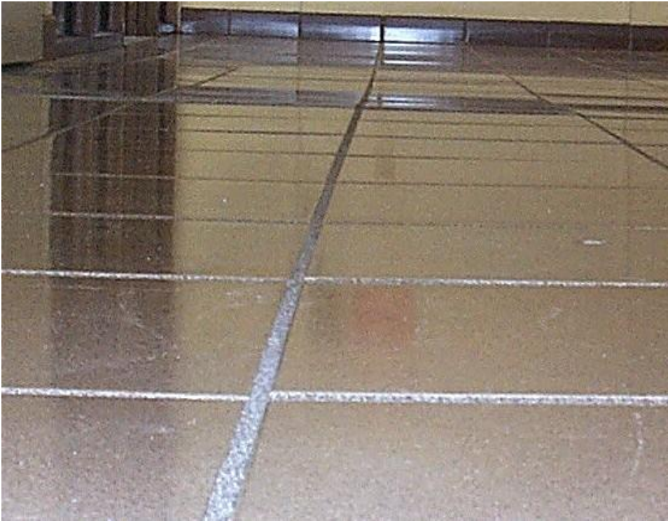
Picture 1-1 – Large format tile highlight imperfections in the substrate.
