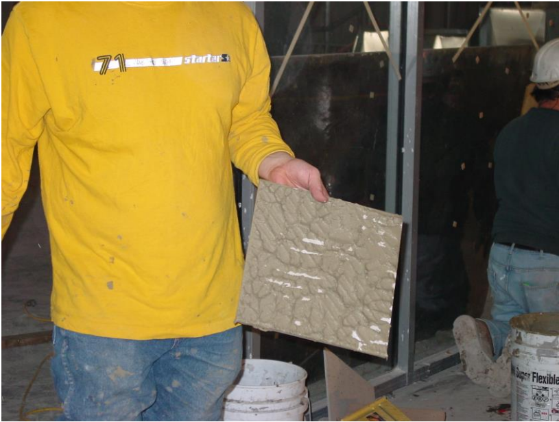
Picture 1.4 – Ceramic tile removed during the installation to verify proper coverage is being attained. Notice the lower right hand corner of the tile is lacking coverage. This will undoubtedly lead to a cracked tile.
